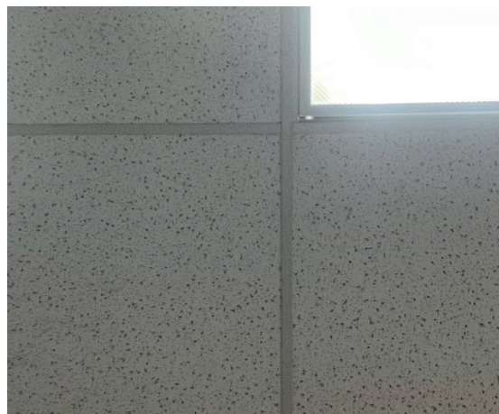
Figure 3. Photo of the Author's Office Ceiling (2022)
